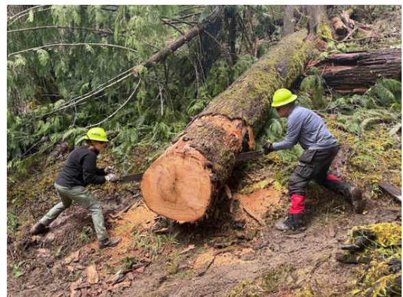
We really didn't have any unexpected difficulties to this project, other than the hillside (and the trail) in this area is wet clay. Extremely slippery. This made safe footing a challenge.
