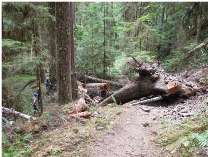
Trunk and rootball pulled downhill.
