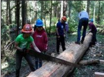
Crew working to create a level walking surface on the top of the log.
