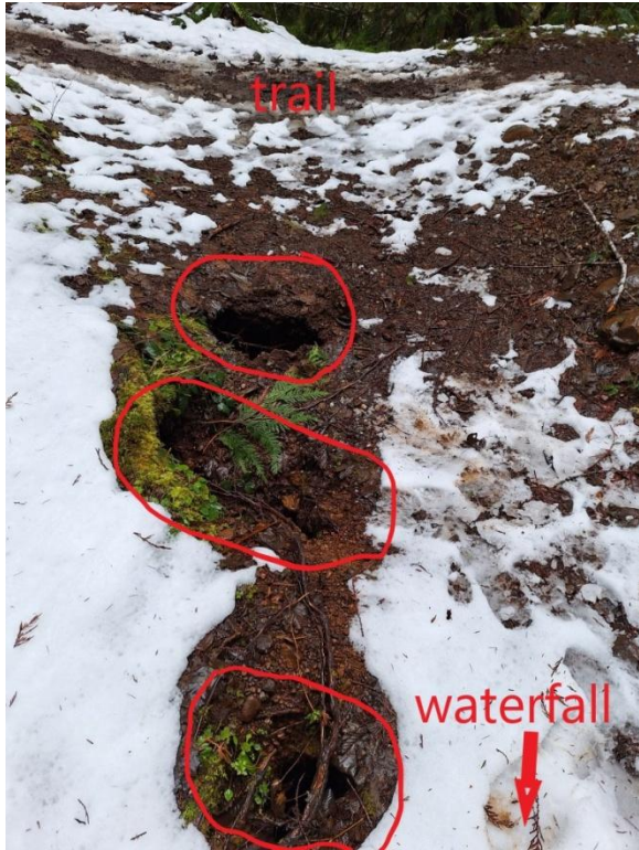
19 Jan 2024: Sinkholes over culvert
